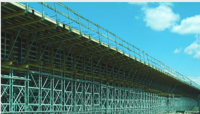
S8 expressway from Wrocław to Łódź (Poland) 961 pcs. of pot bearings 86 pcs. of elastomeric, guide and restraint bearings
